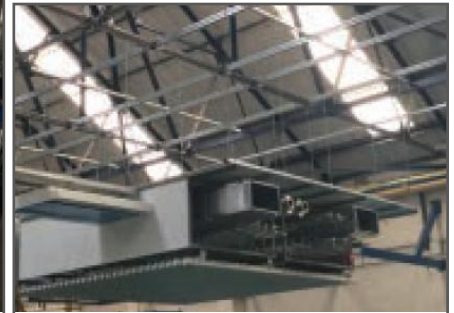
Figure 24: Prefabricated horizontal module with ceiling board, lighting and exit signs
